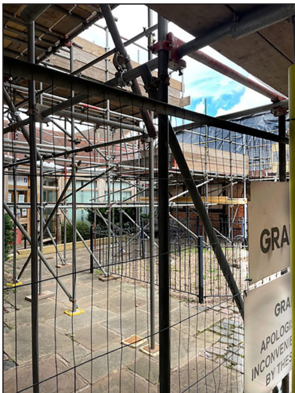
Scaffolding fills the Library Courtyard during the closure, the familiar entrance remaining visible in the background
